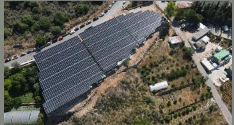
Bellevue Medical Center 750 kWp
