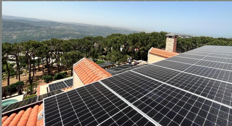
Mar Moussa Villa 22 kWp + 58 kWh
