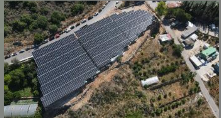
Bellevue Medical Center 750 kWp
