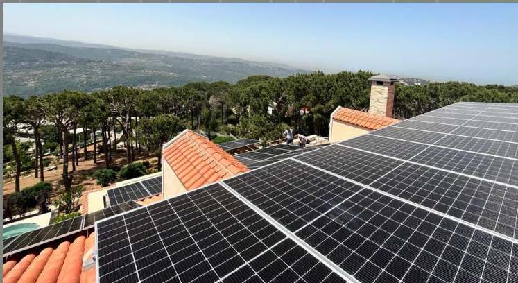
Mar Moussa Villa 22 kWp + 58 kWh
