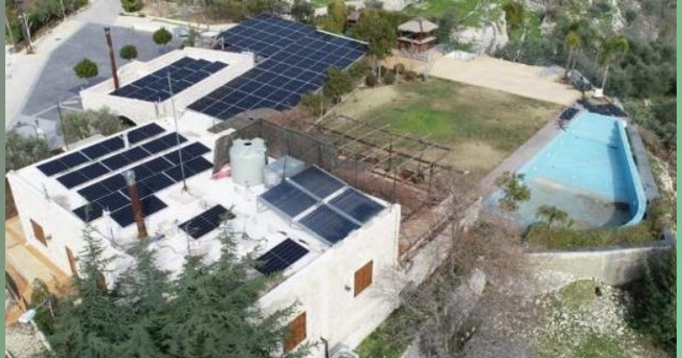
Ghalboun Guesthouse 33 kWp
