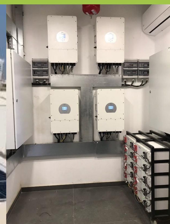
Client: Net Logistics Connection Voltage: 220V
